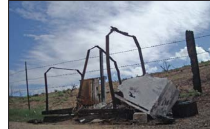
Non-native cell stations were also ruined.
