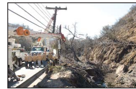
Burned infrastructure took weeks to repair.
