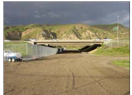
Asphalt has been removed and fencing re-aligned to guide wildlife under the freeway.
